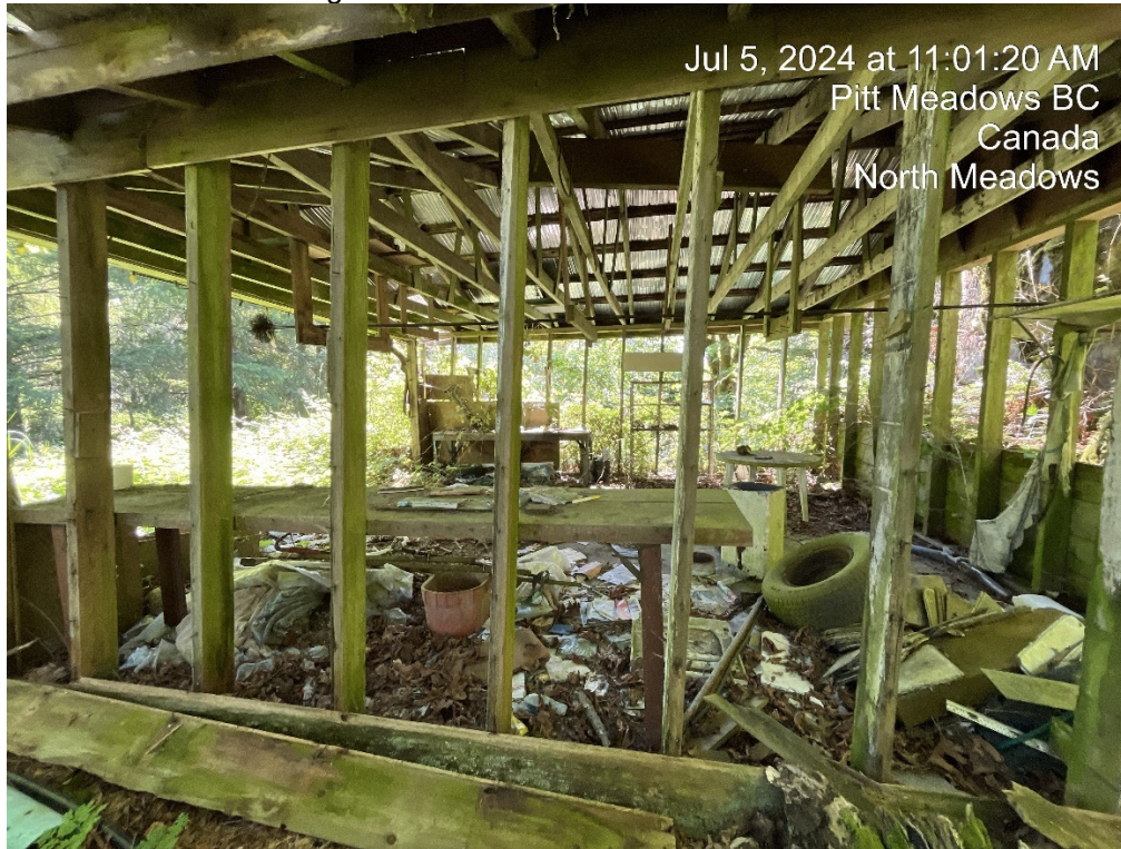
Photo 5. Derelict building at the northwest side of the site.
